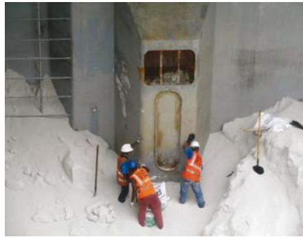
Removing damaged product from cargo hold
