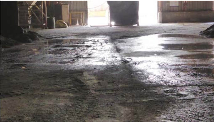
Keep doors closed and remove spilled material immediately.
